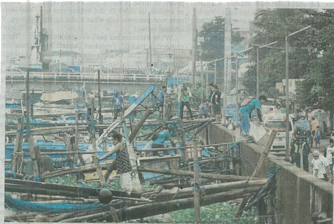
CLEARING OPERATIONS Fishing boats are removed from the stretch of Bangkulasi River between Lapu-Lapu Avenue and C3 Road. —PHOTO COURTESY OF NAVOTAS PIO
